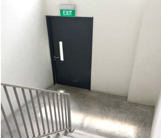
Exit sign placed over the exit door
