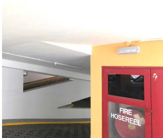
Emergency luminaire at each piece of fire fighting equipment and call point
