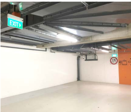
Directional exit signs at each change of direction and in areas where an exit is not readily available
