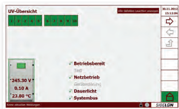
Overview of the connected substations
